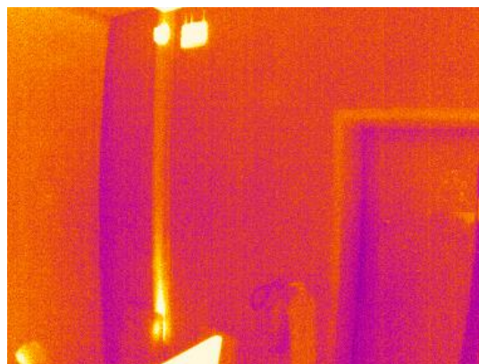
Fig. 9: Optris thermal image cooresponding to the stereo image pair in fig. 7. One can see the warm installation channel and the WiFi device.
