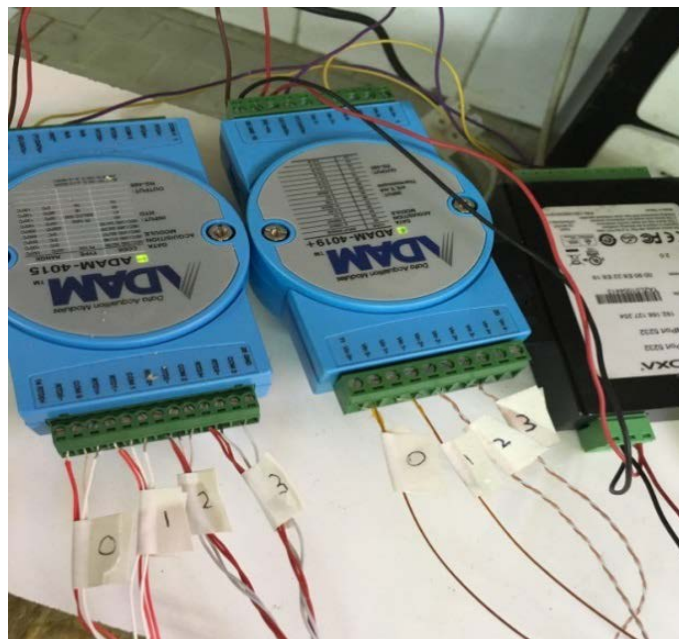
Fig. 2. RTD and TC sensors connected to ADAM modules
