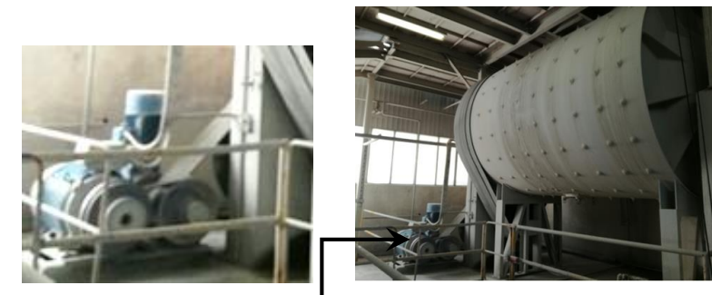
Fig.1. Production station of research with electric drive
